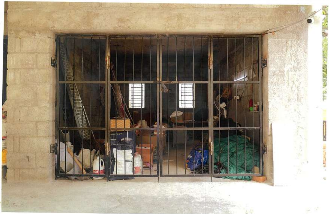
ELECTRICAL TRANSFORMER ROOM (STILT FLOOR)
