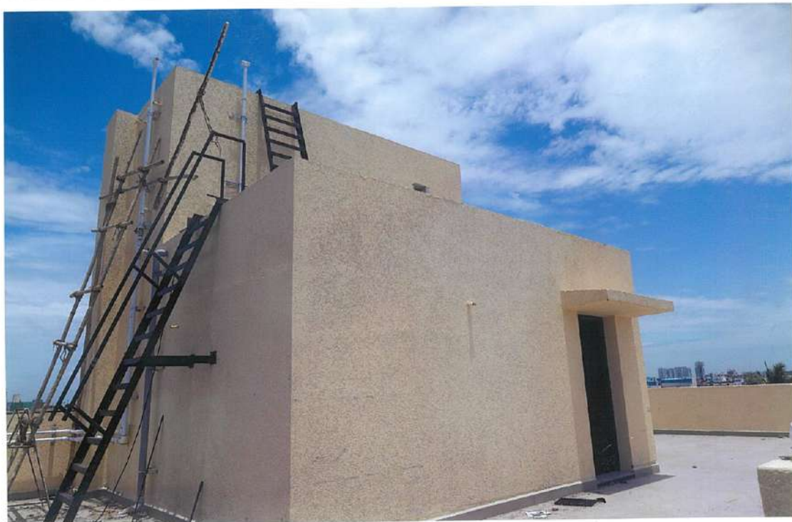
HEAD ROOM LMR & TANK
