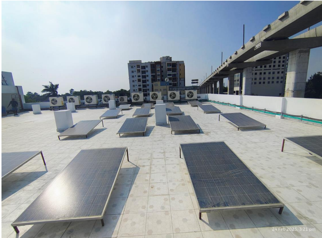
TERRACE FLOOR WITH SOLAR PANELS
