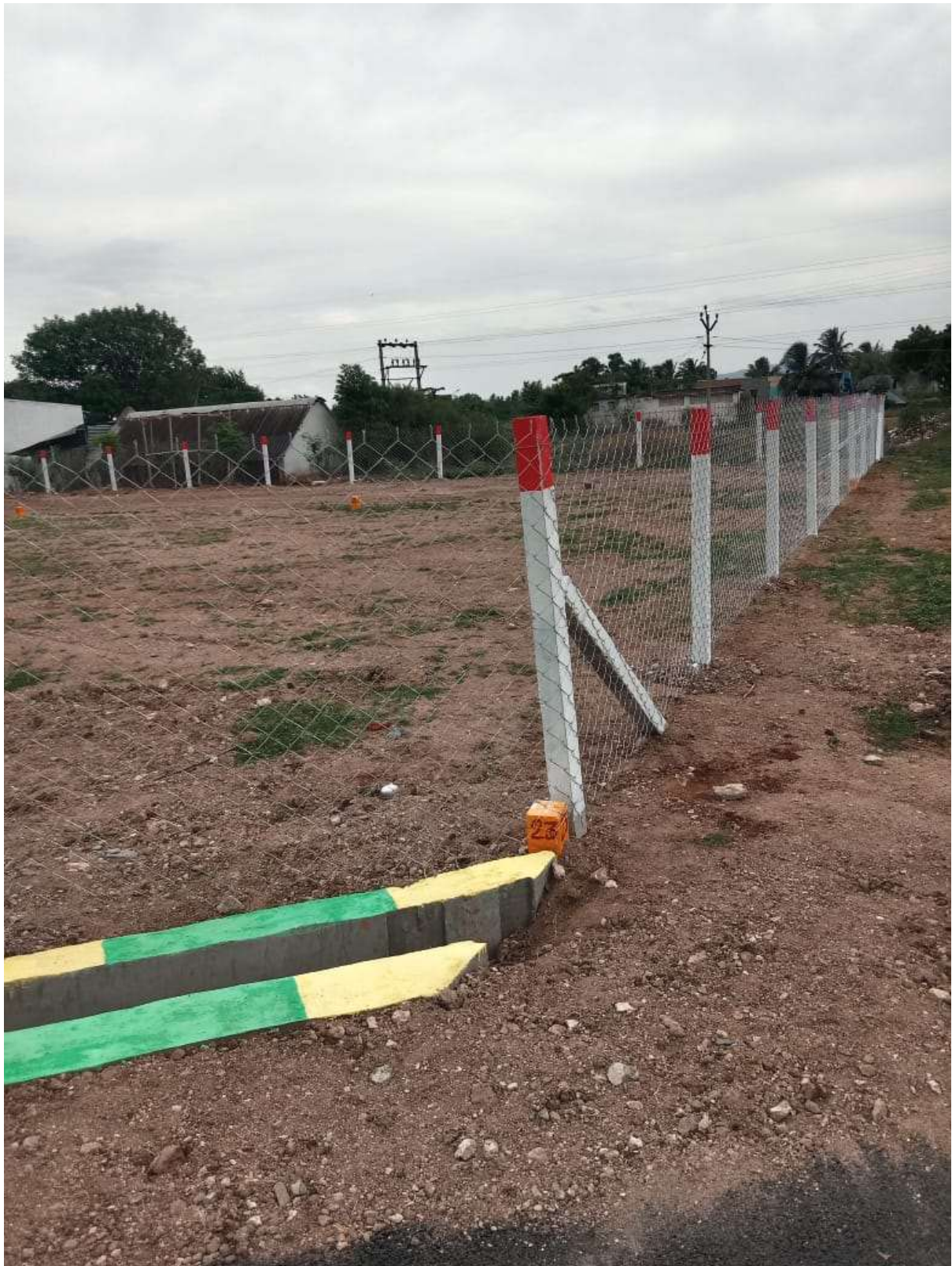
LT line shifting before photos
