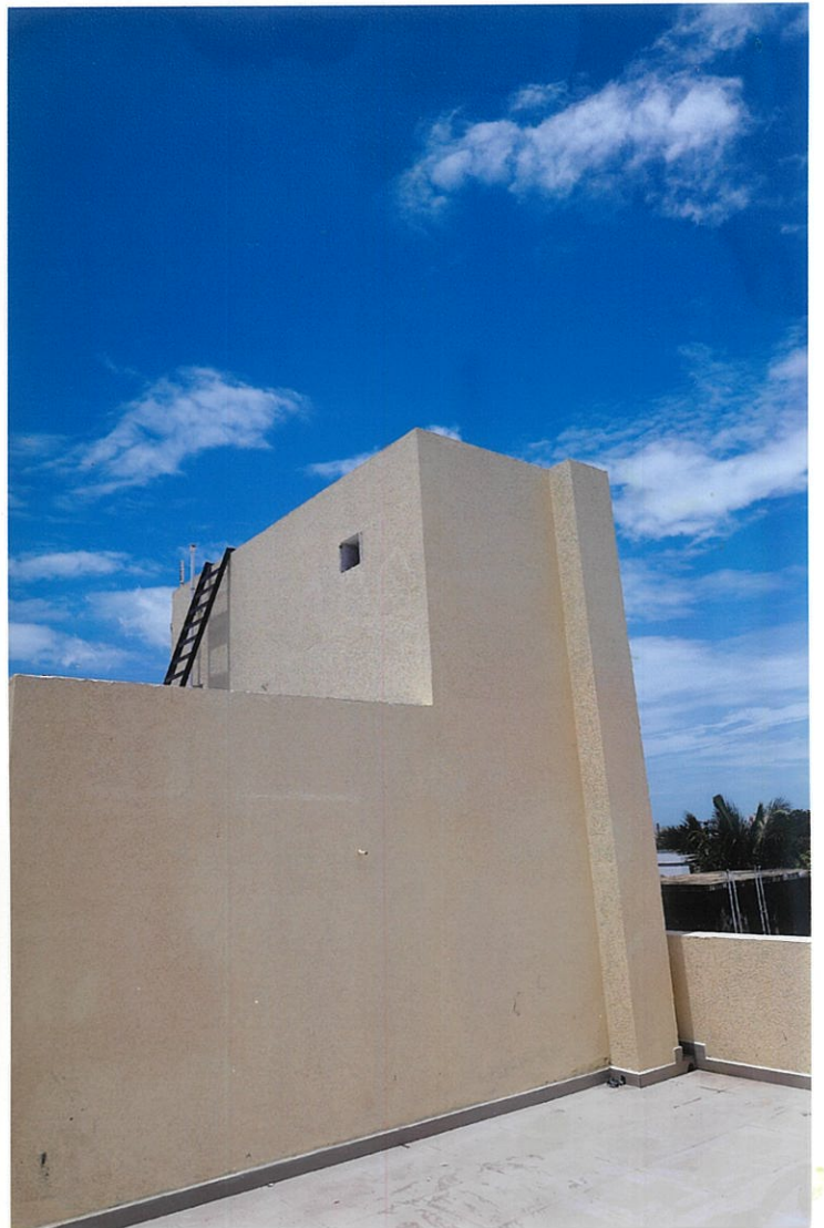
HEAD ROOM LMR TANK
