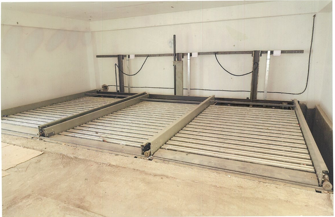
MECHANICAL PARKING IN STILT FLOOR
