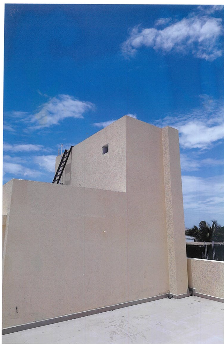
HEAD ROOM MACHINE ROOM WITH TANK
