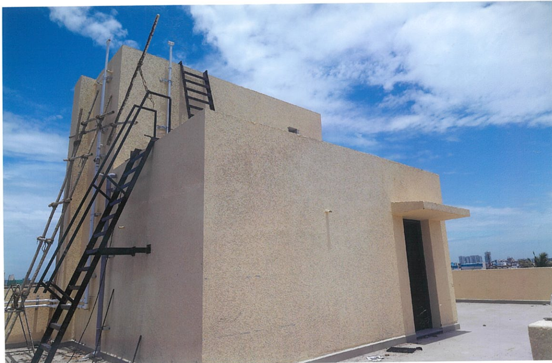
HEAD ROOM LMR & TANK
