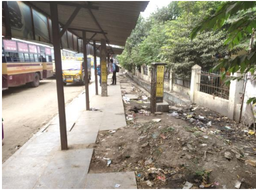
1. Neglected Footpath Facility
