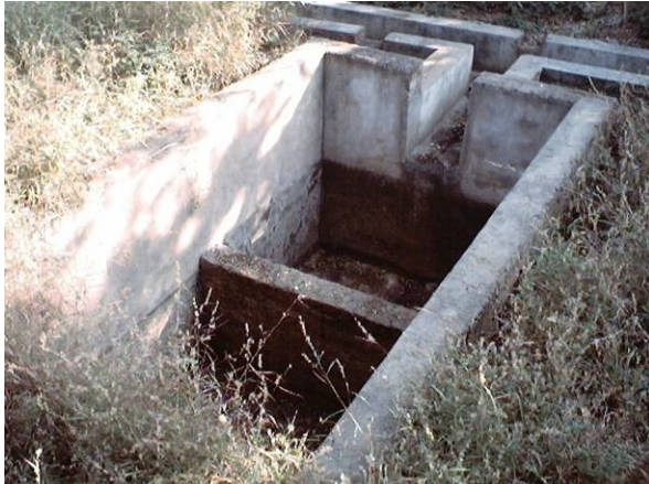
Filter chamber at CLRI for collecting road side run off
