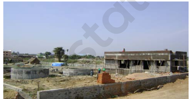
Keelkattalai Main Pumping Station
